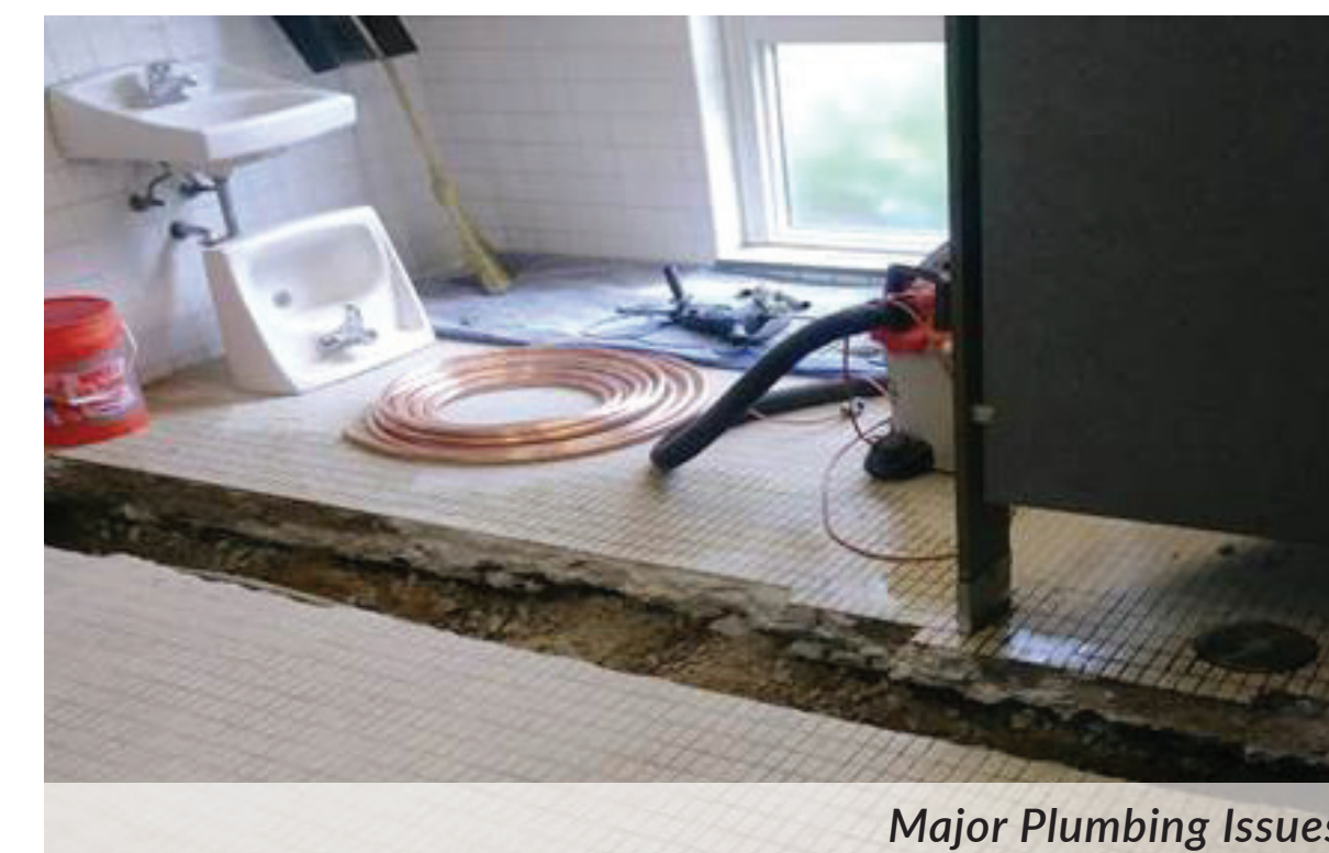
Major Plumbing Issues
