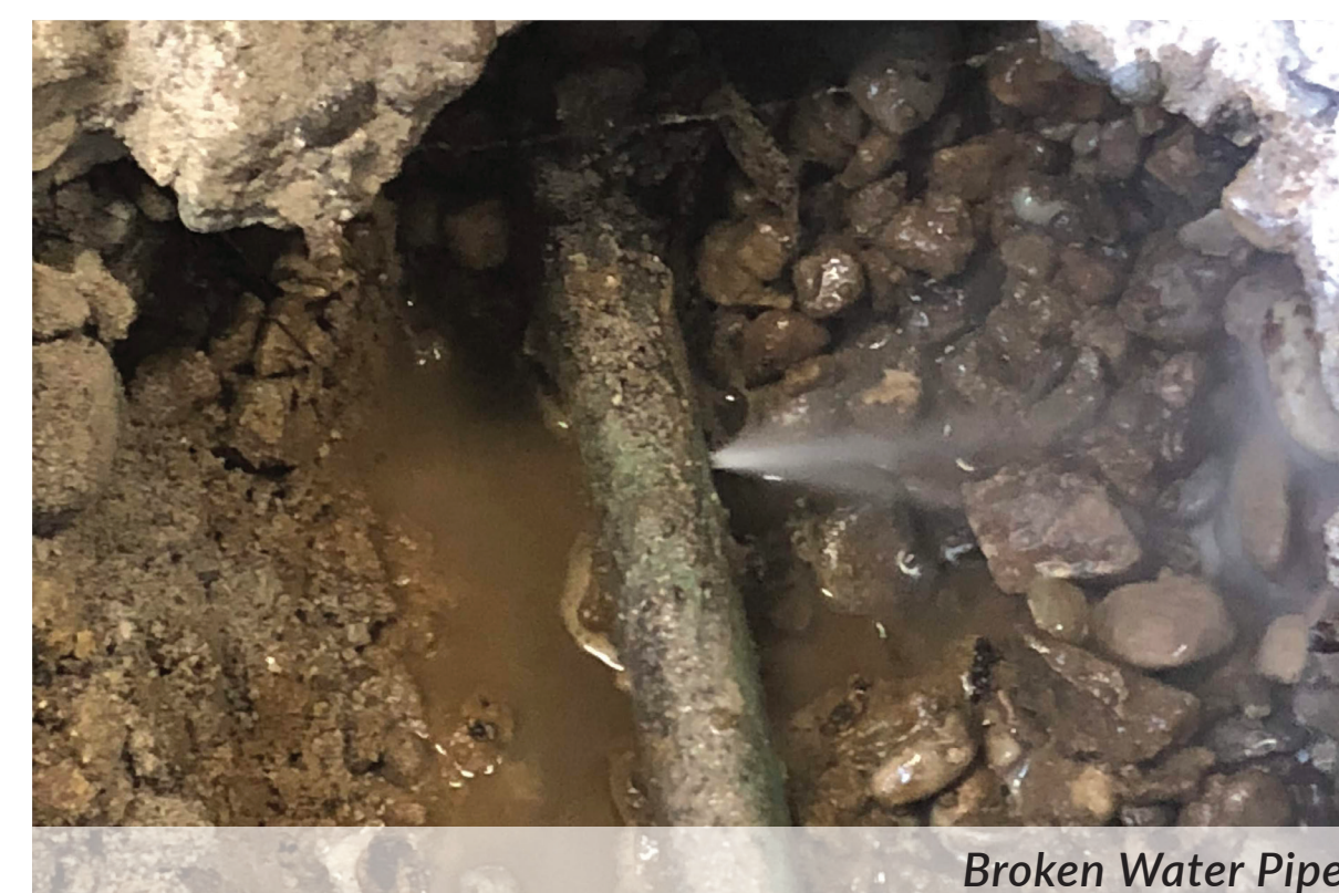
Broken Water Pipe
