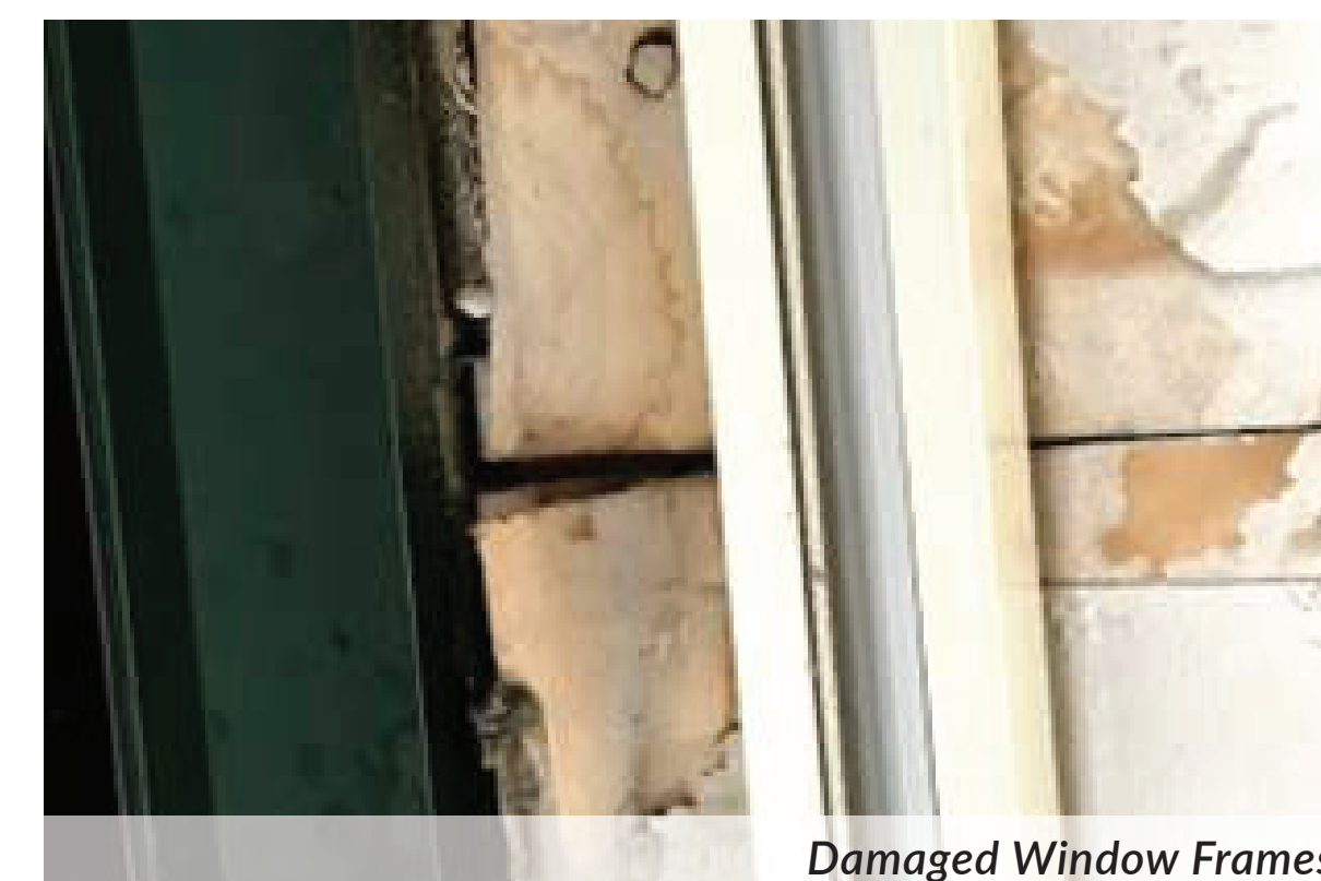
Damaged Window Frames
