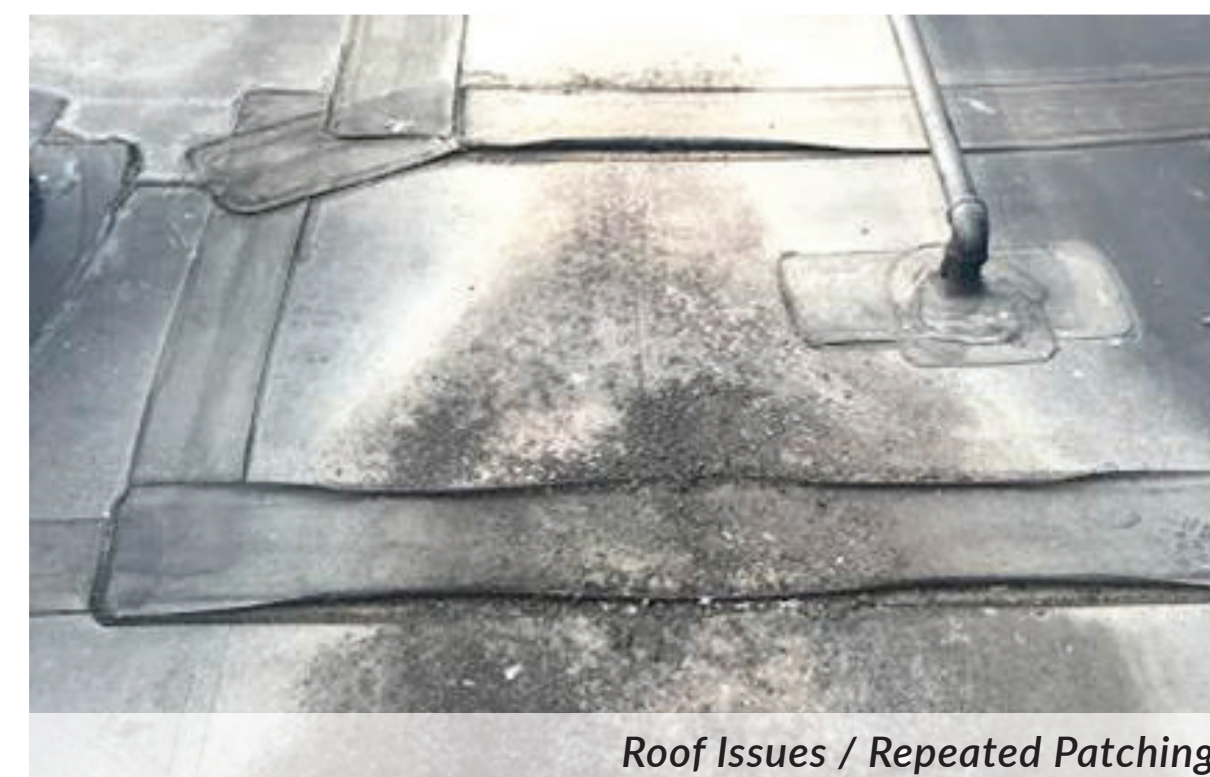
Roof Issues / Repeated Patching
